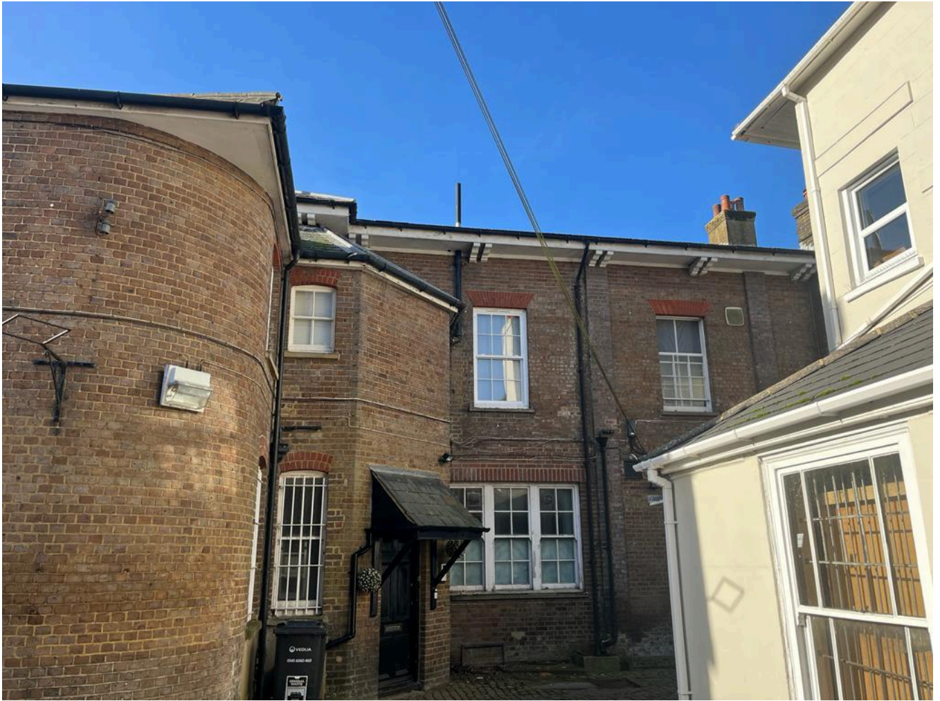
View of top floor Flat 3, and proposed roof area from ground level
