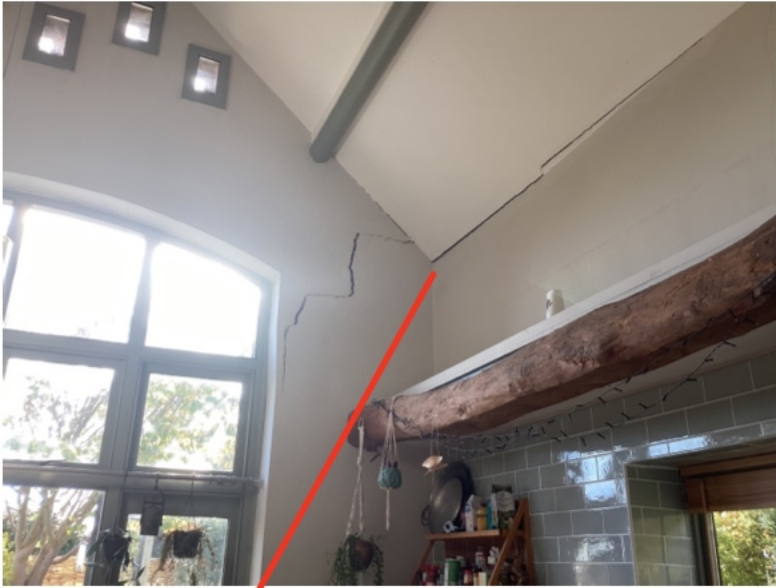
Worst cracking rear left corner
