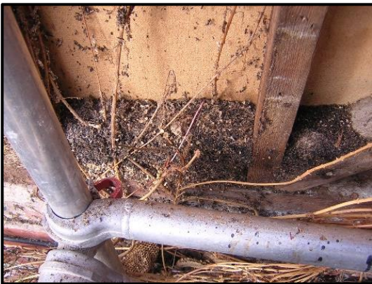
Pipistrelle droppings in exposed wall cavity
