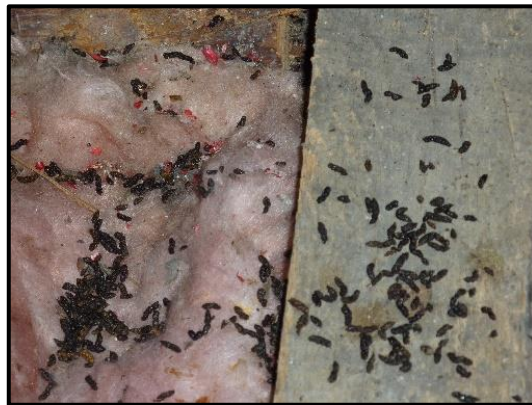
Long-eared bat droppings in roof void
