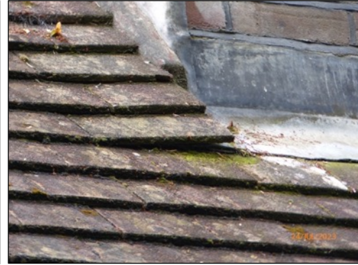
Figure 7: Raised tile on northern elevation by chimney stack.
