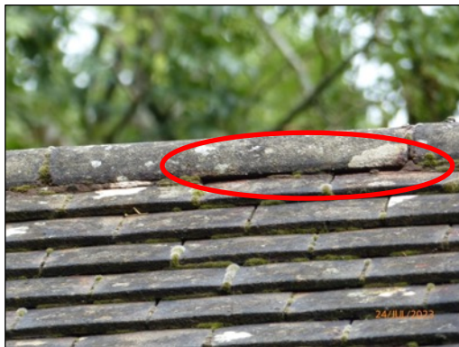
Figure 8: Ridge tile with apparent gap where mortar had dropped out on southern elevation (red oval). Another apparent gap was also present on the northern side.
