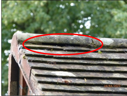
Figure 6: Ridge tile with apparent gap where mortar had dropped out on northern elevation (red oval). Another apparent gap was also present on the southern side.
