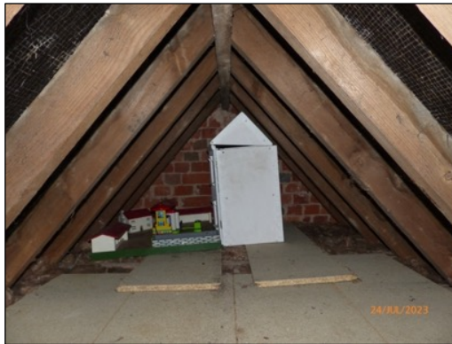
Figure 3: Void 1 – extends in a westerly direction from the central chimney.
