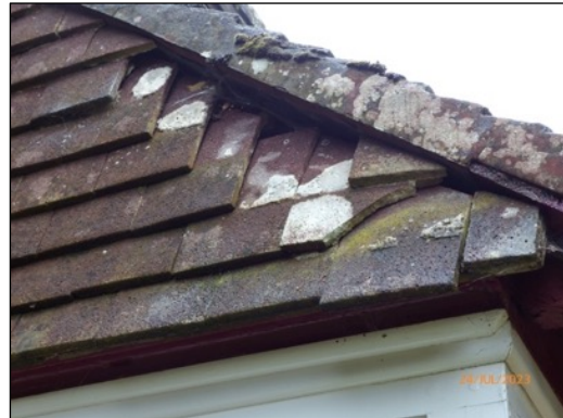
Figure 9: Broken hanging tiles above the porch.
