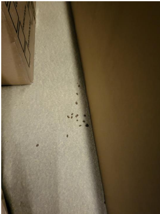
Ref 9: Droppings in roof space
