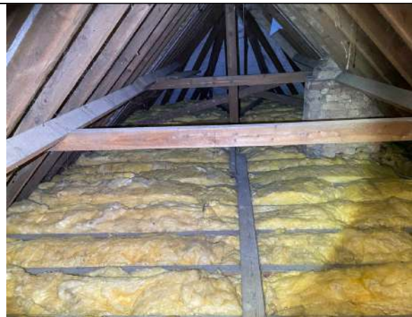
One of the loft voids in B1 Dwelling. It is in an excellent condition, with no bat evidence and no light ingress which could indicate bat access points.
