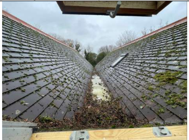
North facing view of the double pitch of B1 Dwelling, taken from the loft void window in the southern void. The roof tiles are in an excellent condition with no gaps.
