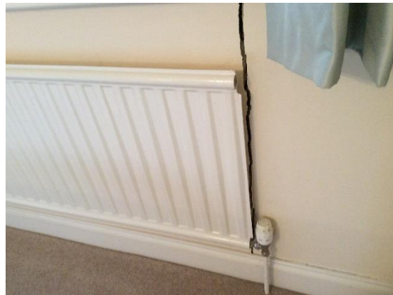
Tapering cracking above and below windows up to 10mm wide.
