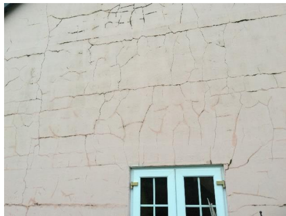
Render in a poor state of repair on gable wall.
