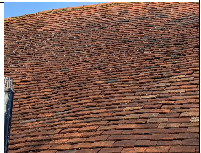
Photograph 6: Gaps beneath roof tiles on the main roof of the house
