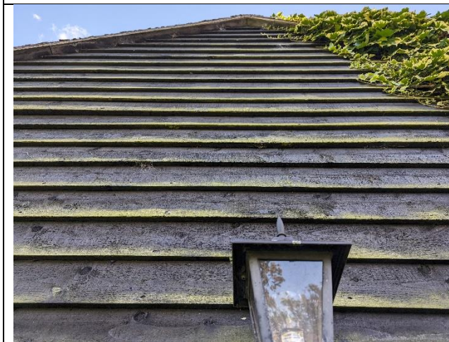
Photograph 3: North gable of the annexe with tight-fitting weatherboarding where extension will tie in
