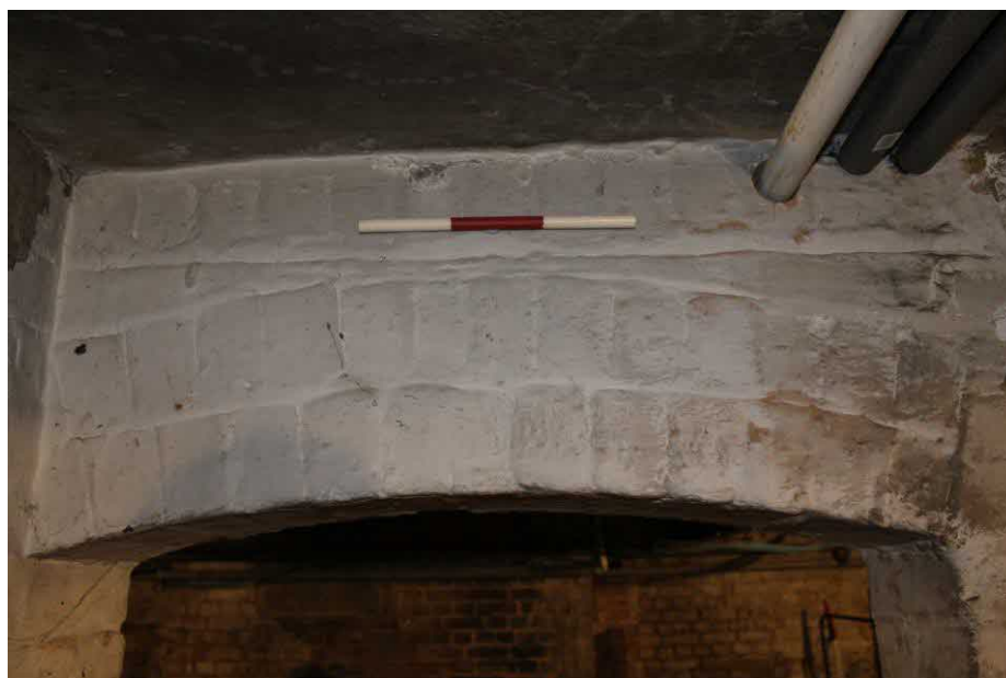
Figure 18 Detail of brick arch above entranceway between Rooms 1 and 3. Soldier course of bricks visible at top of wall. Photograph taken facing south.
