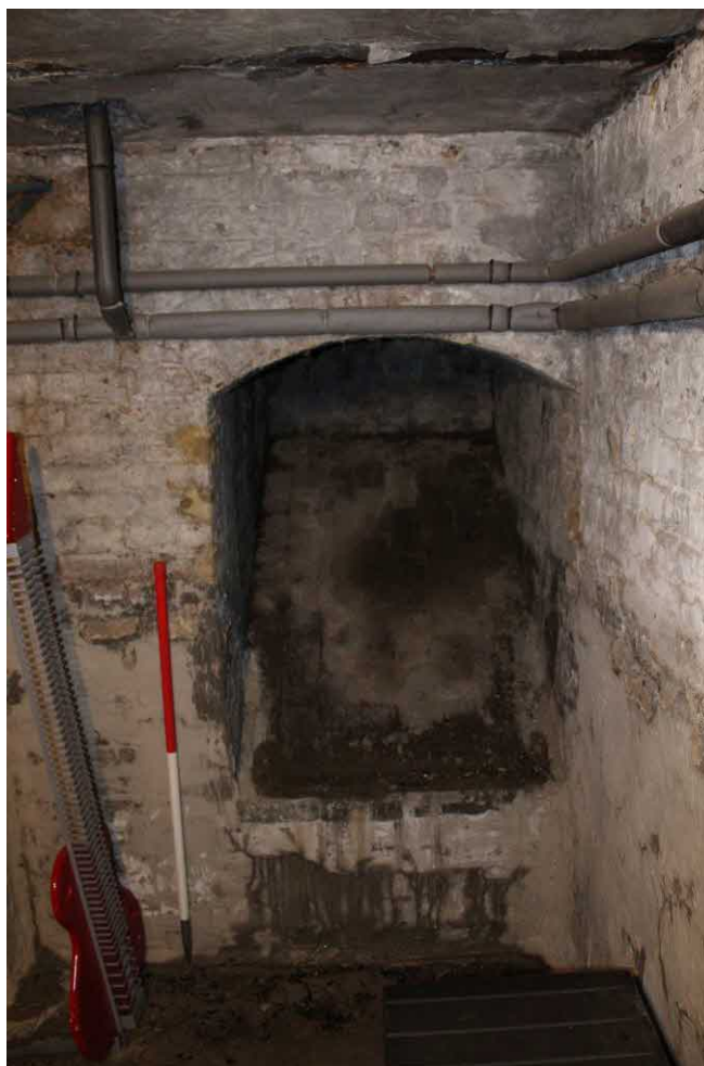
Figure 22 Detail of coal chute on southern elevation of Room 1. Photograph taken facing south.
