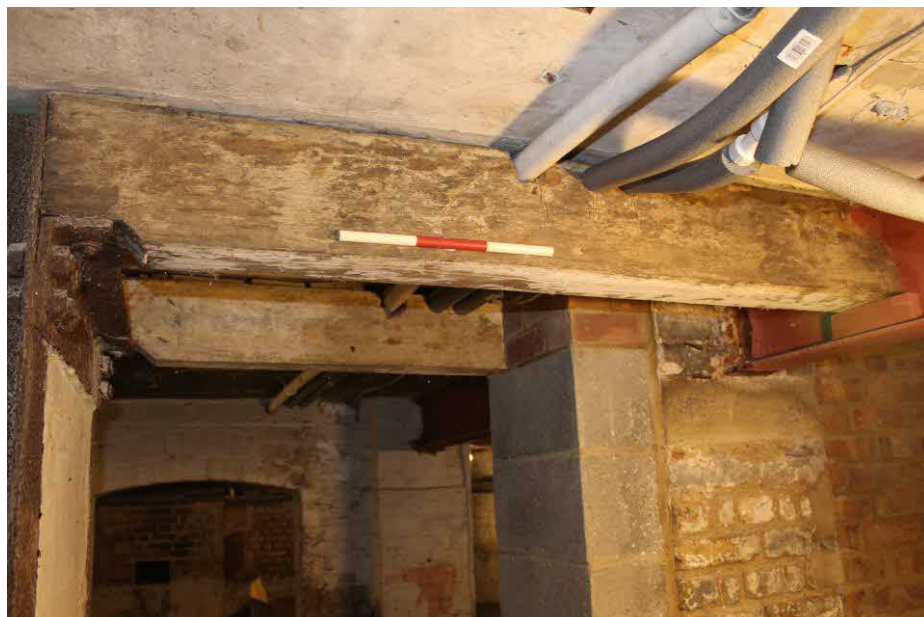
Figure 34 Timber beam supported on ironwork to left of frame and modern girder to right. Concrete blocks added to original brick pillar visible behind. Photograph taken facing south.
