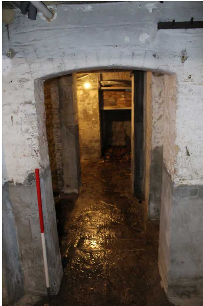
Figure 25 Original arched entrance between Room 1 and Room 3. Water ingress into basement also visible.
