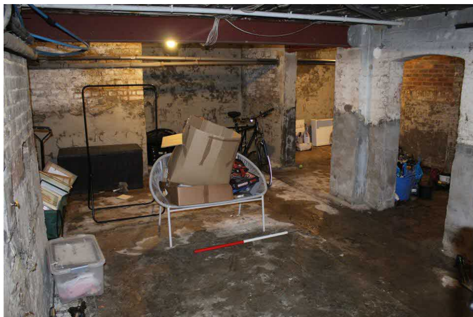
Figure 26 Western end of Room 1. Entrance into Room 2 visible in background. Original brick-arched entrance into Room 3 visible to right of frame. Photograph taken facing north-west.
