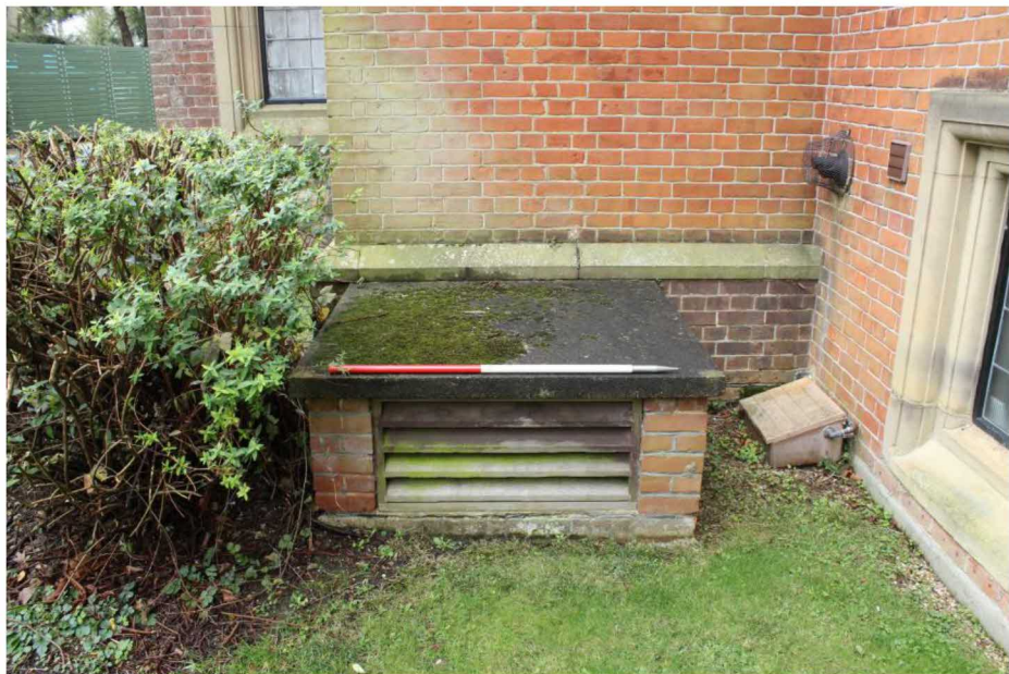
Figure 13 Detail of vent above coal chute on southern elevation of 4 Hadham Hall. Photograph taken facing north.
