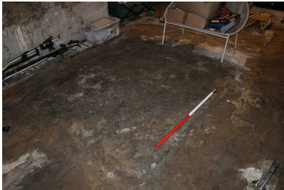
Figure 29 Detail of raised concrete area in Room 1. Photograph taken facing south-west.
