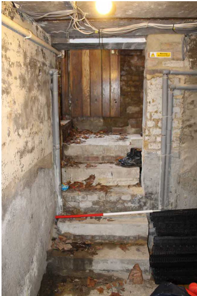
Figure 35 Modern access into basement from converted coal chute. Photograph taken facing north.
