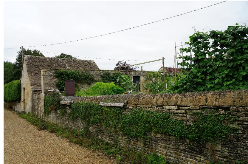
Fig.7 Boundary walls to no's 14 & 15, and tall garden wall in front of 'The Smithy'
