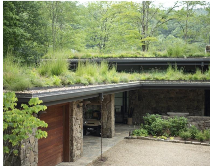
Fig.24 Green roof planted with native species to improve habitat and contribute to sustainable drainage strategy
