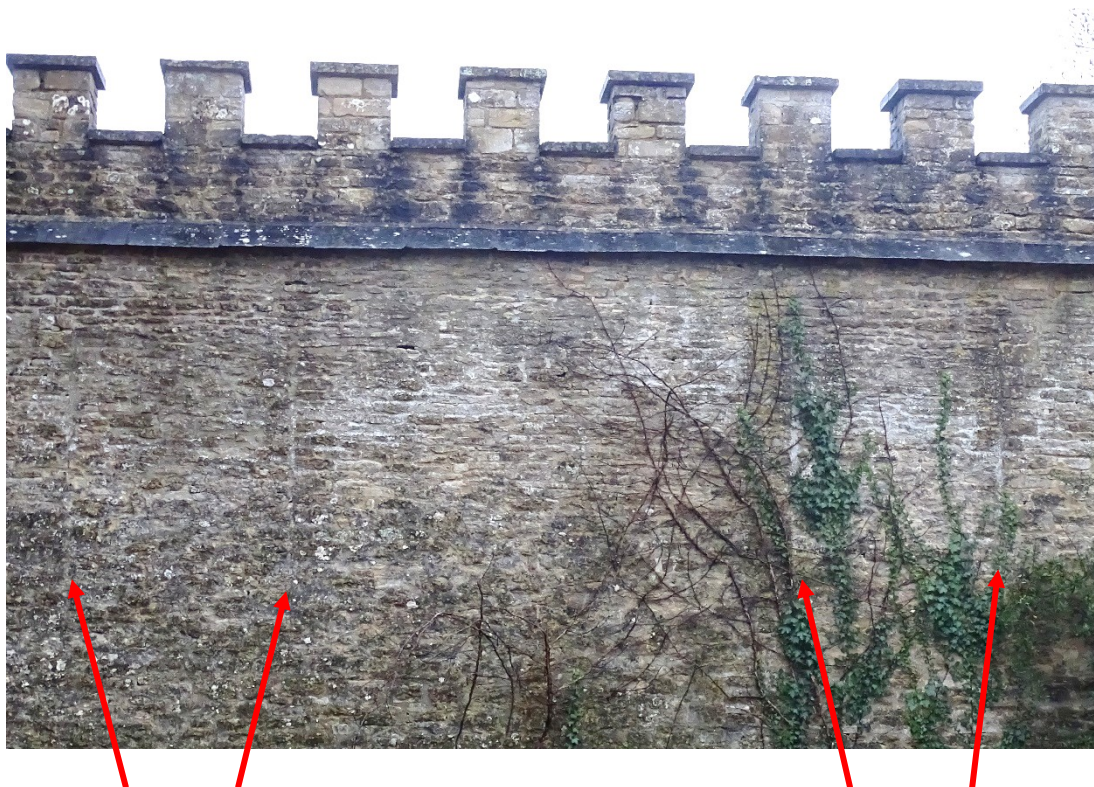
Vertical joints, windows 2 and 3, indicated by red arrows
