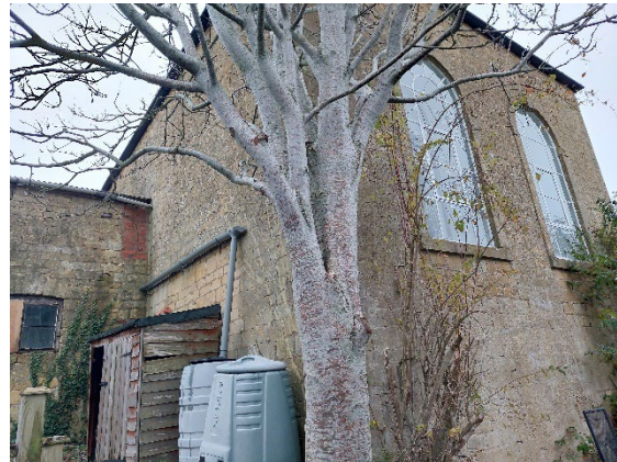
Figure 4.11 – Rear (south) elevation of Village Hall. Showing connected outbuilding of Hainault House.
