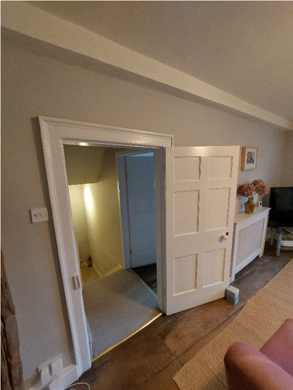
Figure 4.6 – First floor Georgian paned door with raised surround, one of several internal historic fenestration surviving.
