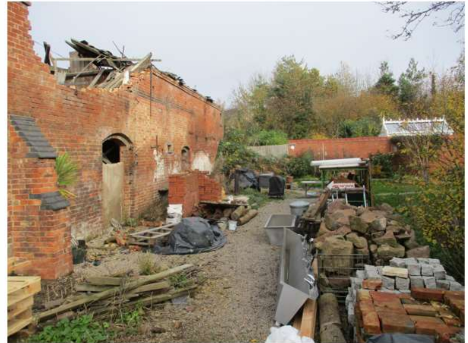
Photo No.4: Facing north showing the rear (eastern) face of the dilapidated barn
