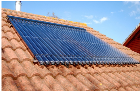
Figure 6: Typical solar thermal panel
