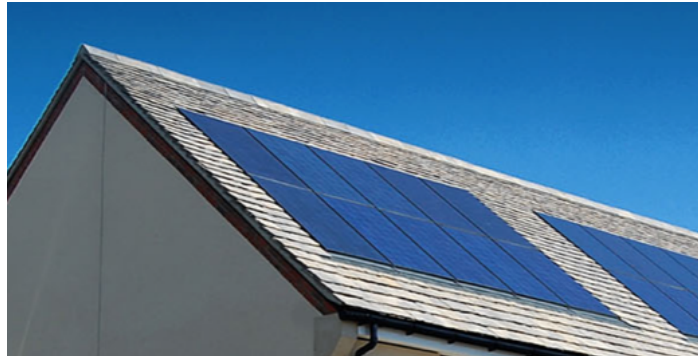
Figure 9: Typical PV installation to pitched roof
