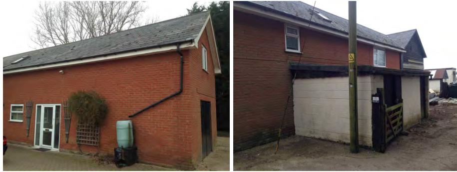
Eastern and western faces of the eastern annex (also showing the flat-roofed extension on the eastern side)
