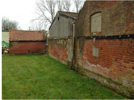
Northern face of asbestos clad extension opposite the pond. Also showing the north face of the western annex (closet) and Outbuilding 1
