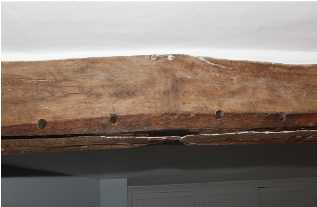
Illus. 8. A detail of the centre of the tie-beam in illustration 6 showing the narrow gap between the brace mortices and two pegs for the crown-post above (figure 11). The timber bears a 'dagaz' symbol scratched by the carpenter to indicate the timber's best surface, which faces the high end of the hall. Although the timber has been cleaned it has escaped the usual sand-blasting and preserves its original surface with unusually fine deposits of soot from an open hearth. Similar deposits are visible on the rafters.
