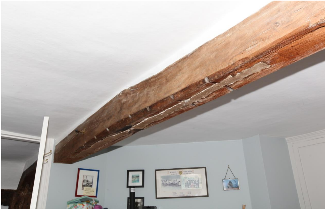
Illus. 7. The centre of the tie-beam in illustration 6 contains plaster-filled pegged mortices for the missing arch-braces of the open truss. These braces rose from matching mortices in the wall posts and formed a high and relatively flat Tudor arch in the fashion of the late-15 th and early-16 th centuries.
