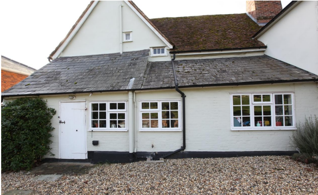
Illus. 5. The step in the slate roof of the rear lean-to is not matched by any obvious break in its external brickwork and probably relates to the lower eaves of the medieval hall on the right (rather than indicating two phases of construction). The structure was added in or about the 1840s as part of William Synnott's remodelling. The windows are late-20 th century replacements and the 19 th century door with characterful pintle hinges on the left also appears to interrupt the brickwork. The partly removed internal partitions suggest the original door occupied the position of the central window.
