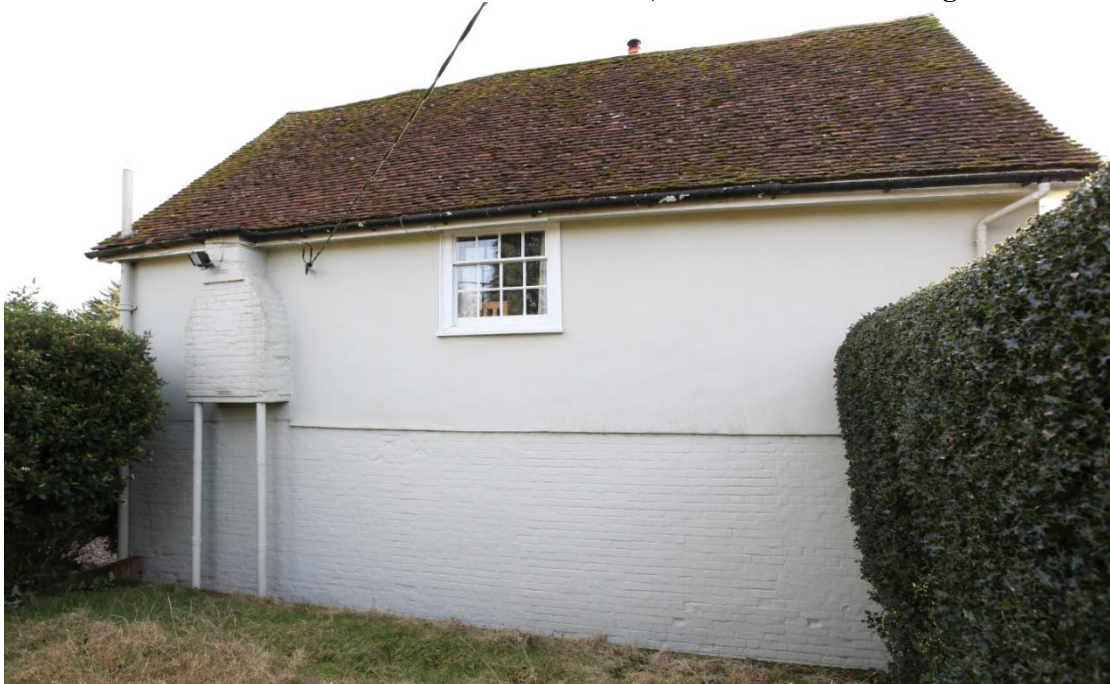
Illus. 2. The northern side of the parlour wing showing the Flemish Bond brickwork of its lower storey and a first-floor chimney curiously supported by iron posts. There is no evidence of a fireplace in the brickwork beneath, and it is unclear whether the chimney was designed in this way or was truncated when the lower wall was rebuilt.
