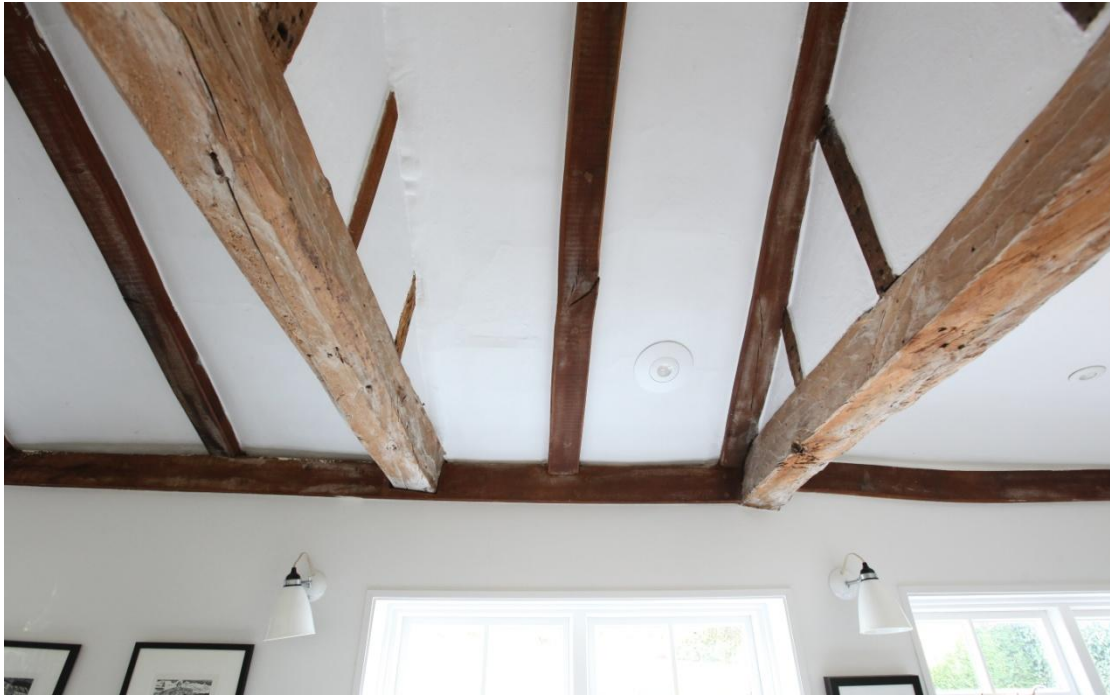
Illus. 17. The narrow gap between the original tie-beams in the centre of the lean-to suggests that a rear door occupied the position of the 20 th century window. Nail holes and scars in the undersides of both timbers indicate the missing studs of two partitions forming a narrow passage that probably linked the external door to the medieval cross-passage (assuming the latter was undershot – i.e. beneath the ceiling of the service wing rather than within the open hall). The exposed rafters and roof-plate are modern.
