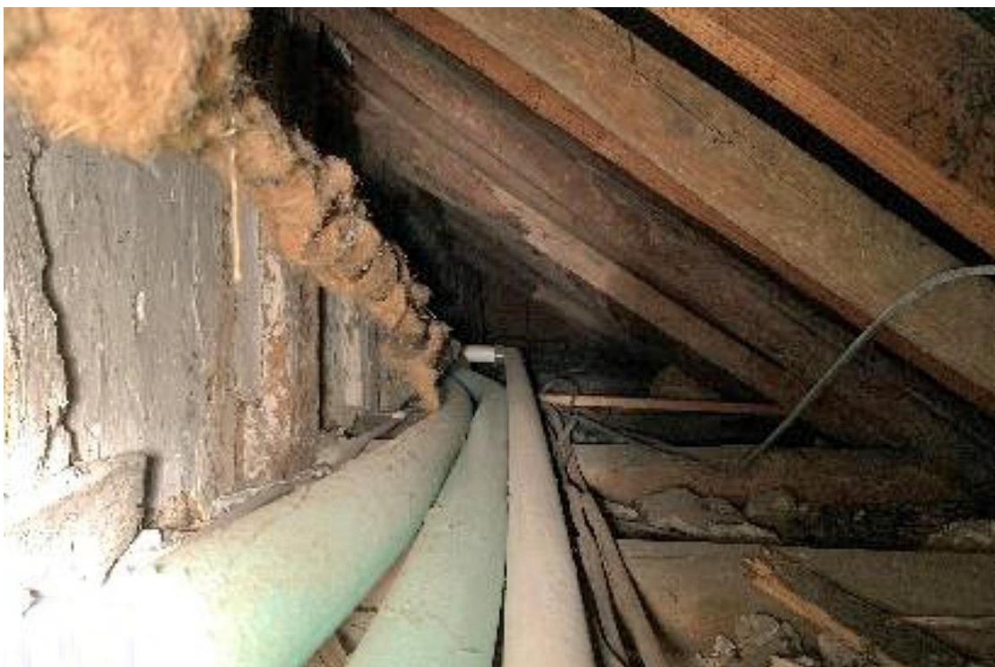
Illus. 16. The rafters above the ceiling in illustration 14, with the whitewashed studs of the hall on the left. As in illustration 15, the roughly hewn rafters and ceiling joists in the rear are typical of the 19 th century while the softwood examples are replacements.
