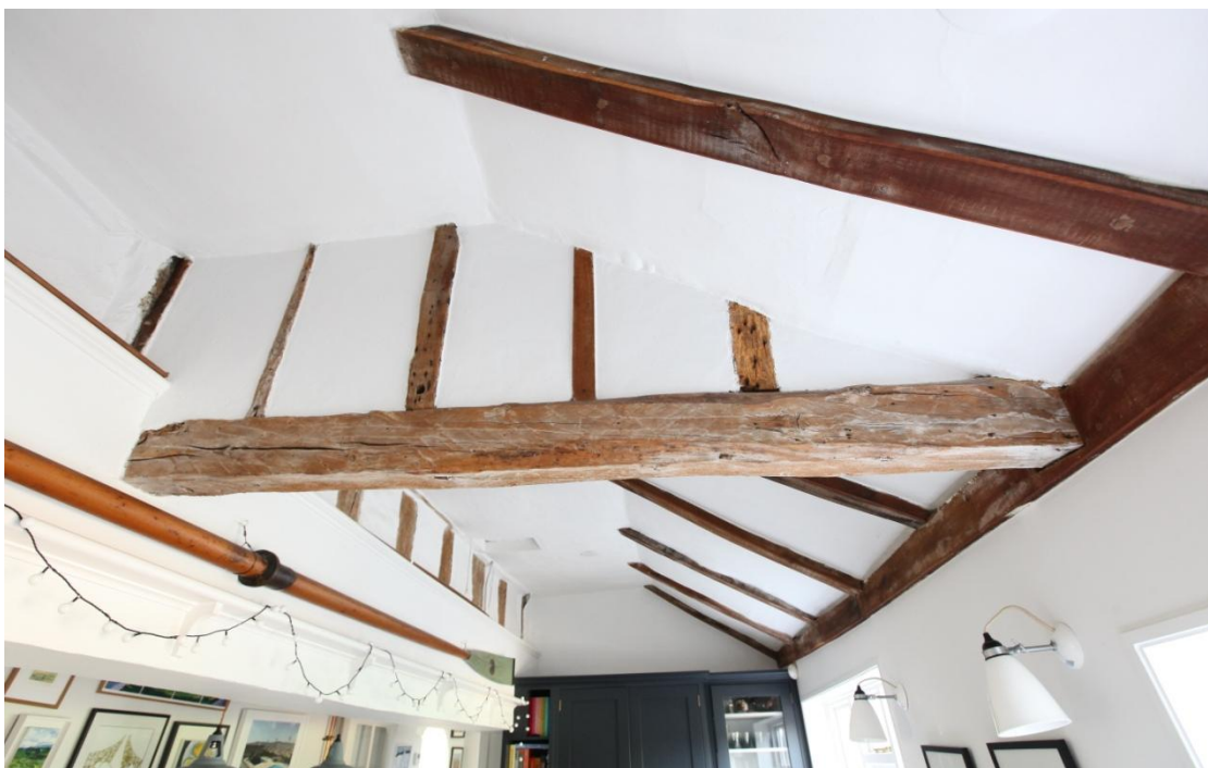
Illus. 12. A detail of the tie-beam in illustration 11, as seen from the south-east. The timber was formerly hidden by plaster, as indicated by the scars of laths nailed to its sides, and nails for the missing studs of a ground-floor partition are visible in its underside. The false roof-plate and rafters to the right bear modern saw marks.
