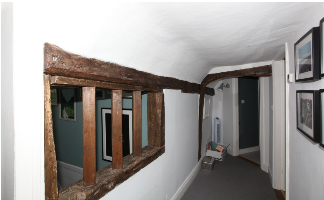
Illus. 6. The first-floor corridor to the rear of the former open hall, showing the tie-beam of the open truss carrying the crown post in figure 11 in the rear. The roof-plate on the left contains the shutter rebate and mullion mortices of a tall high-end window that lit and ventilated the hall, but this is now overlapped by the stair turret and its diamond mullions are modern replicas.
