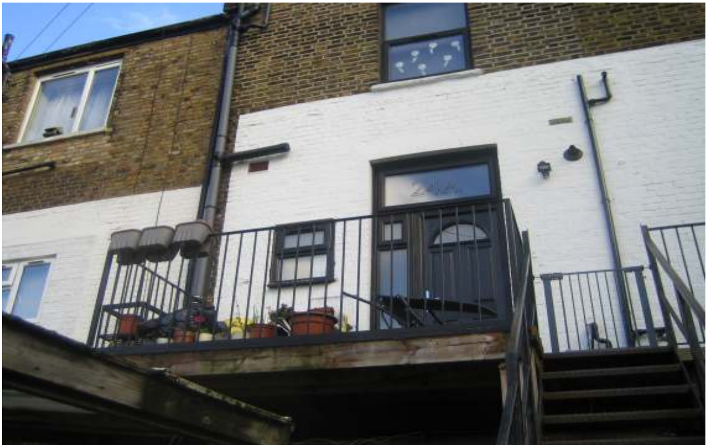
Photo shows the existing rear residential access metal stairs / door to the existing split level flat.
