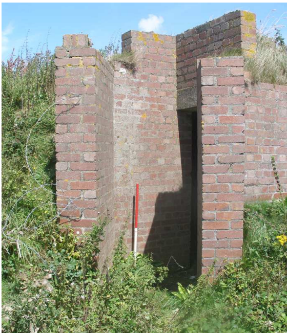
Plate 3 Site 9 brick-built blast protection for Stanton air raid shelter at centre of fighter pen looking east
