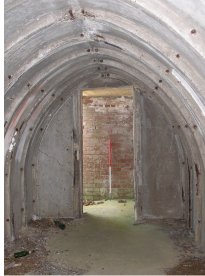
Plate 4 Site 9 Interior of Stanton air raid shelter at centre of fighter pen looking northeast
