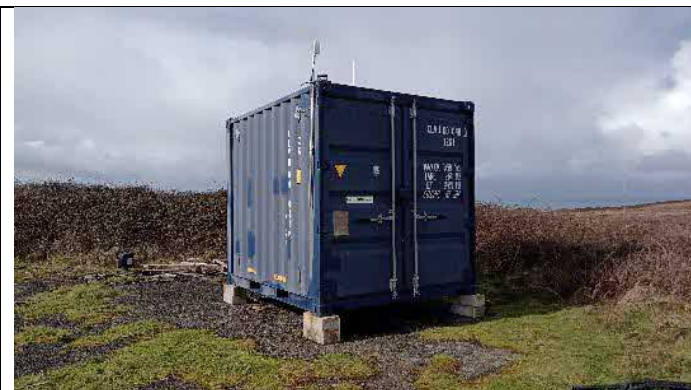
Fig 1 Shipping container signal box
