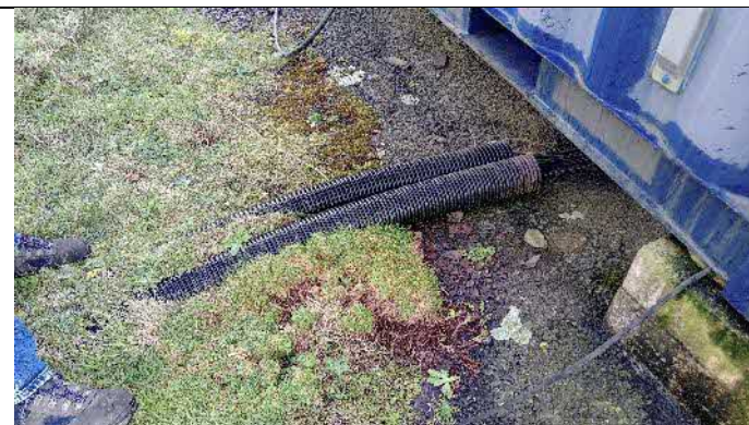
Fig 2 original conduit and cables with vegetation growth
