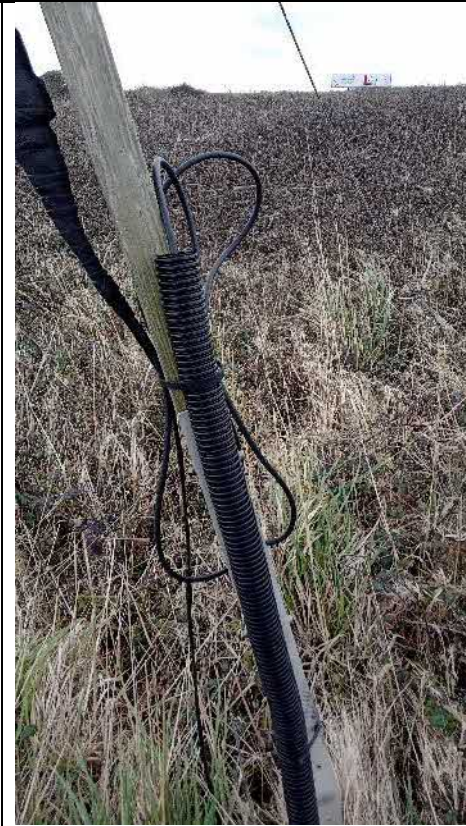
Fig 9 cable and conduit feeding off antenna
