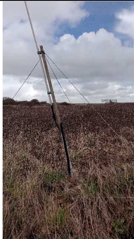
Fig 9 Existing post with antenna
