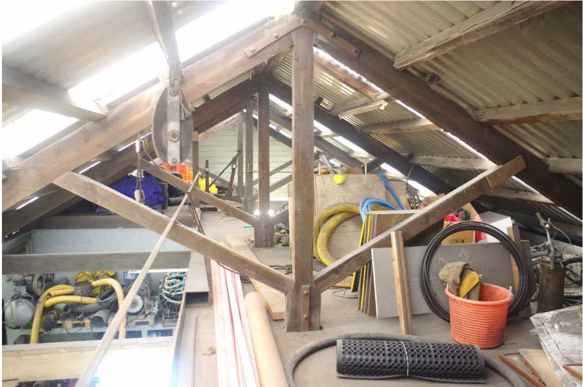
Fig 24 King post trusses dating to c1880 inside the Penwith Marine Services building (Site 34).
