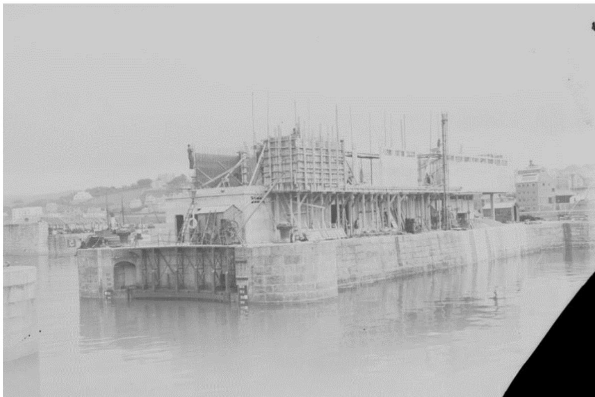
Fig 15 The Rank warehouse building under construction in 1937 © Morrabb Library Ref: IND 16PG 069.
