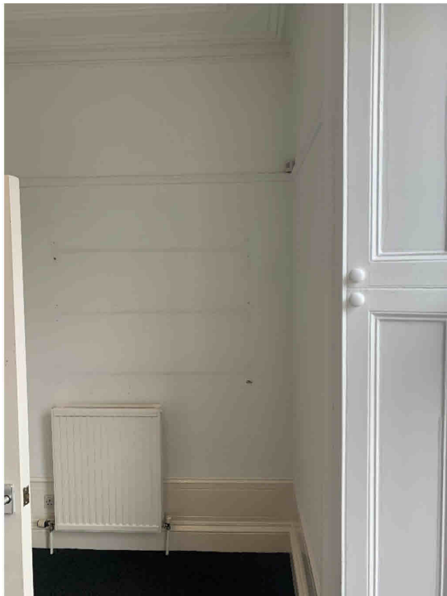
Ground floor skirtings, cornice, picture rail and timber panelling all to be retained
