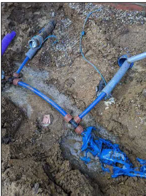
Photograph 1 – Water pipes laid within a trench in the ground. The brown stripe on the pipework is visible, indicating barrier pipework.
