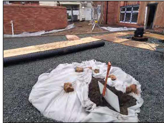
Photograph 6 – View across all three positions showing surplus geotextile membrane at the surface after being lapped through the base of the planters.
