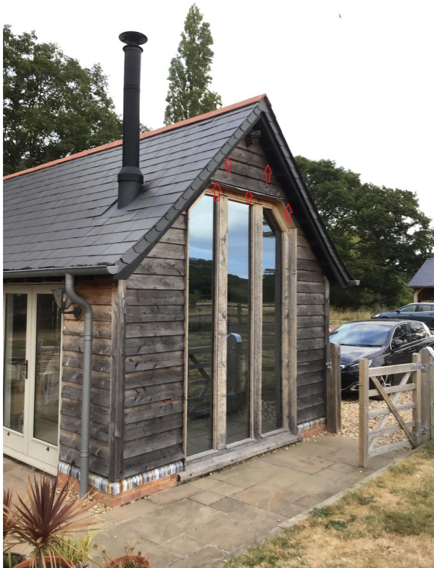
Fig 2. Southern elevation looking north. Red arrow indicate potential access points for bats.
