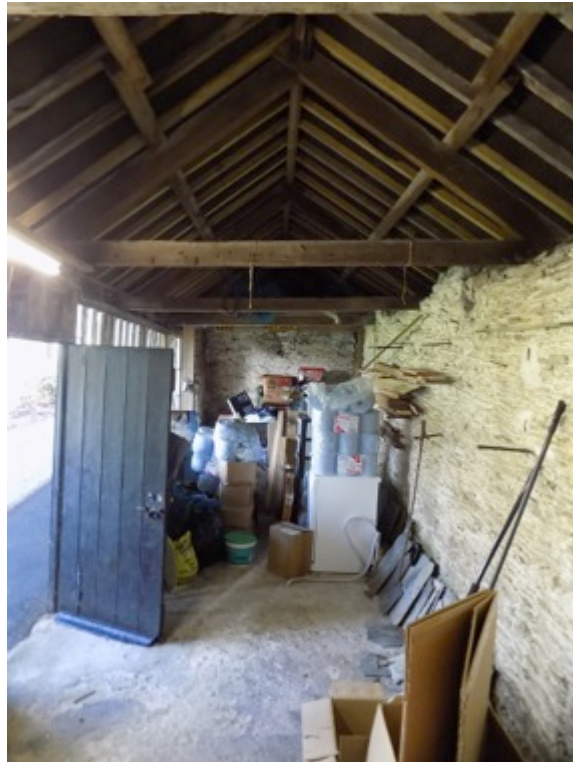
Photo 5. Outbuilding interior with A framed collar trusses, rubble stone and timber frame walling.
