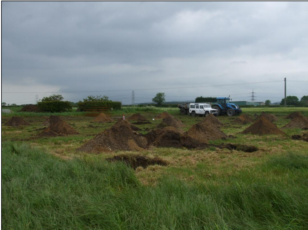
Plate 3: Stanchion pits excavated around the perimeter of, and across the footprint of, Agricultural Building A. Facing north-east.
