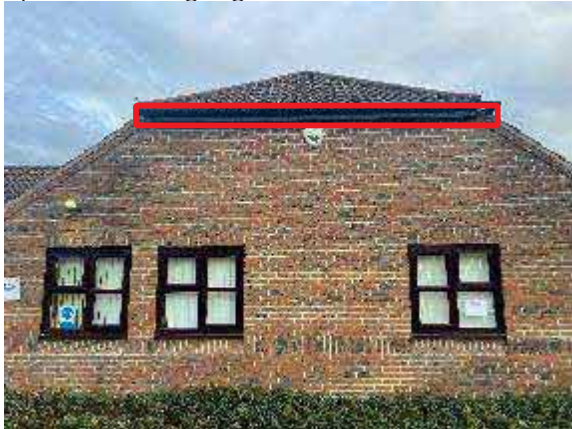
Photo 1 – southern elevation of building 1, open soffits highlighted.
