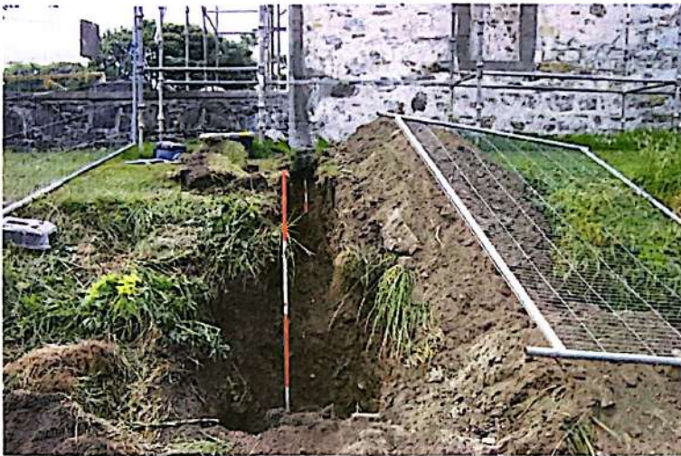
Photograph 7 – shows Soakaway ‘A’, looking W. Only a depth required for drainage was excavated and no attempt was made to ascertain the original ditch profile.
