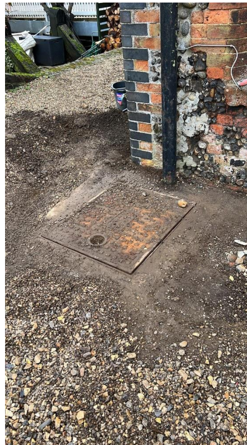
Above Reduced ground level : Exposed Manhole Cover
