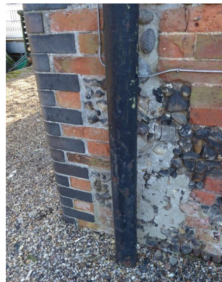
Above Areas of badly repaired mortar to knapped flint to be repaired using heritage lime mortar
