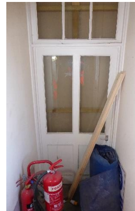
Left Corridor wall accommodation side. Full height glazed partition with access door.
