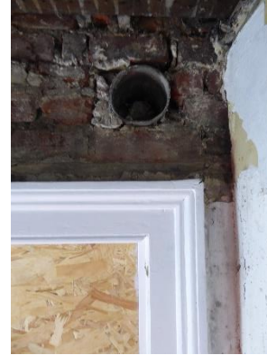
Above Photo 4. Showing existing vent.
