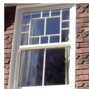
Detailed glazing bar pattern in keeping with the original Revival style of the early 1900s.
