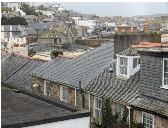
Photo 5. Showing the south facing slope of the roof with a number of missing and slipped slates being visible
