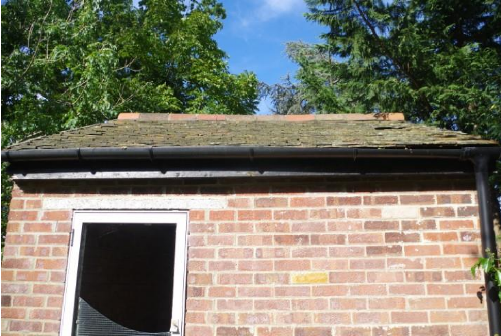
Photo 11. The brick shed was checked but had no signs of bats. If signs of bats are found and works are proposed to shed then a SQE will need to be on call if demolition/ re-roofing is proposed.
