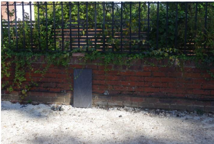
Photo 14. Access track to 29A and 29B Beech Hill, has concrete and brick wall boundary. This will need to be broken out for planting of trees and native hedgerow. See Landscape plan by LandVision (October 2023) for details.
