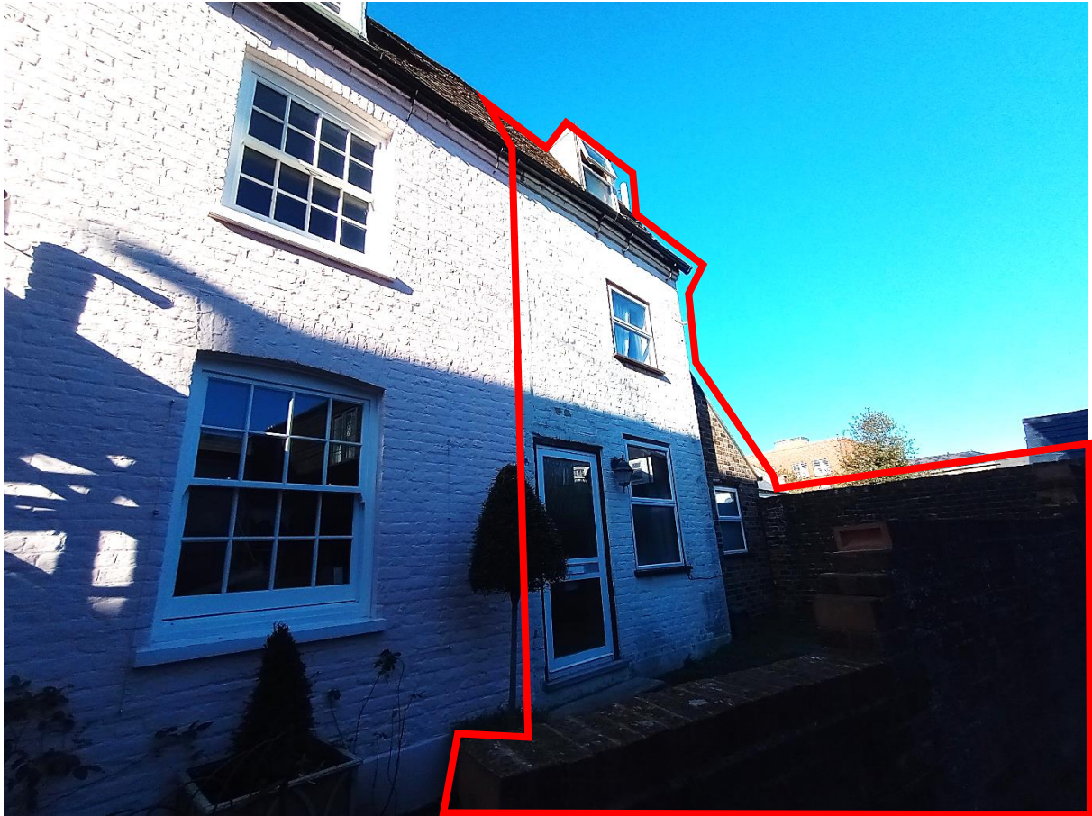
Figure 3 Braunton extension has windows and doors that do not match. The brick perimeter wall is failing structurally
