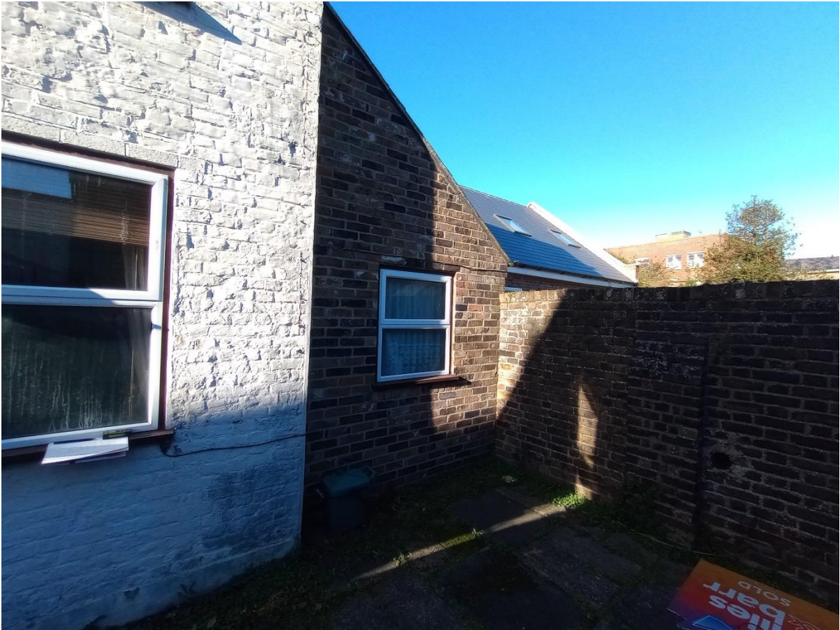
Figure 5 A side extension has been added to Braunton in the late 20th century that sits along the party boundary.
