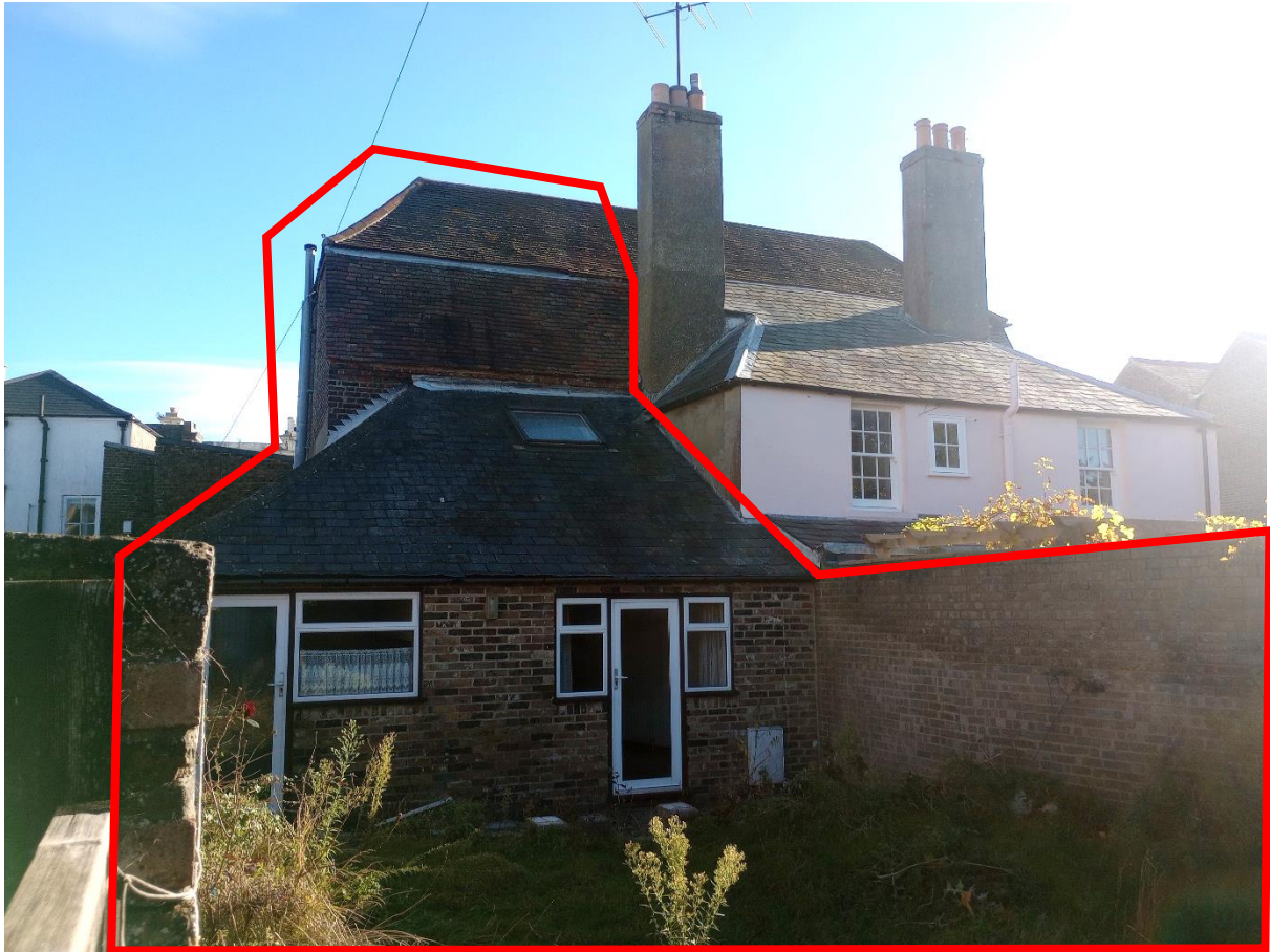
Figure 6 Rear Elevation of Branton. Prospect House is to the right. Braunton was extended in the mid 20th century to the side and rear. Head heights are insufficient.
