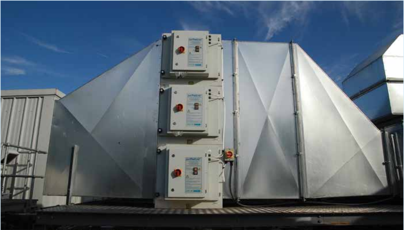
3 ESP Units Stacked in modular formation
