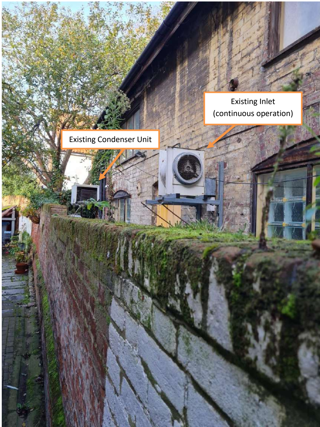
Figure D3 – Photo from private footpath facing The Site boundary showing existing kitchen plant located in external storage area (placement of Measurement Position).
