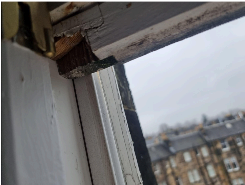
Deteriorating tenon joints.
