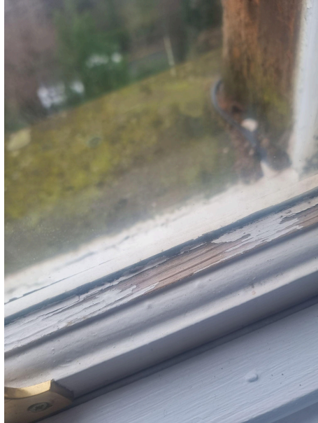
Internal bare wood of the previously replaced window is soft pine wood and is already showing signs of deterioration.
