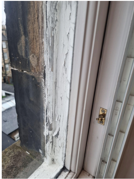
Deteriorating and rotting woodwork to external casement.
