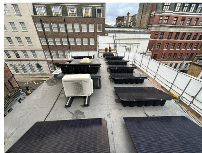
PHOTOGRAPH OF INSTALLED PV UNITS & AIR CONDITIONING UNIT ON FLAT ROOF
