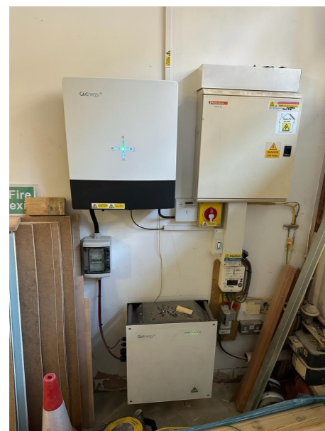
PHOTOGRAPH OF INSTALLED SOLAR BATTERY AND CONVERTER IN GROUND FLOOR GARAGE SPACE
