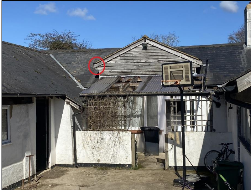
Photograph 5: Emergence point shown in red
