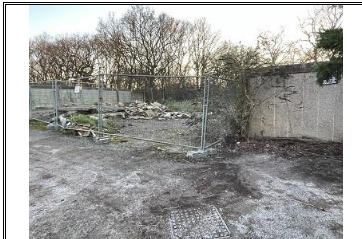
Photo OE/1702/1058/R1/P03 – View of northern area of the site and original garage blocks.
