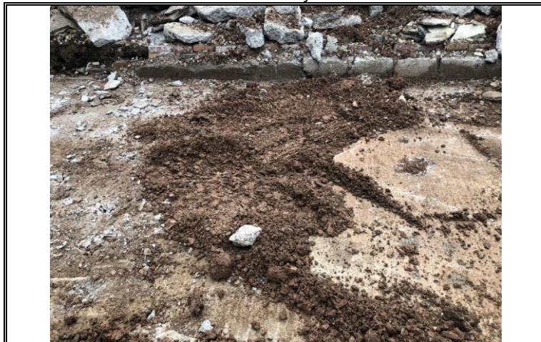
Photo OE/1702/1058/R1/P 21 – Excavated area beneath original slabs to central section of the garages.
