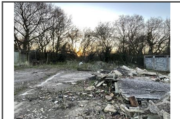
Photo OE/1702/1058/R1/P06 – Centre of concrete slab between original garage blocks – looking east to west.
