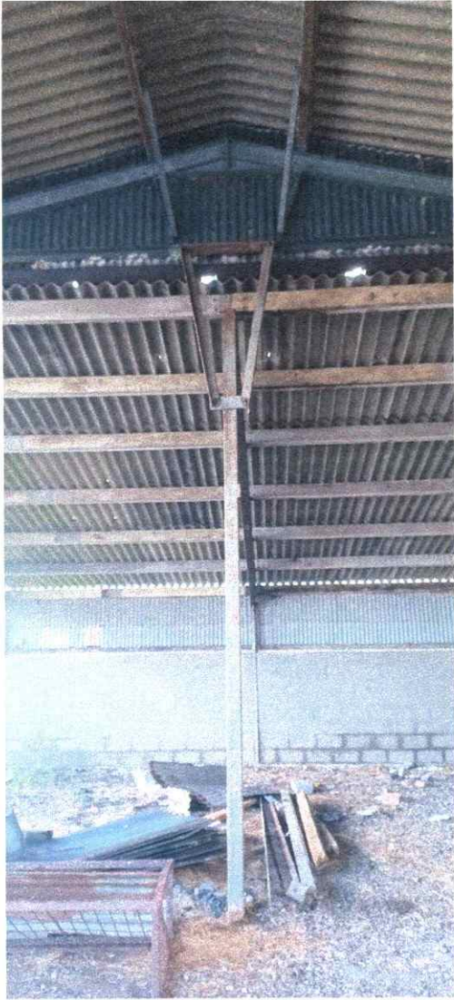
Lean to structure to east elevation. Roof structure in timber and steel shown to be in good condition.
