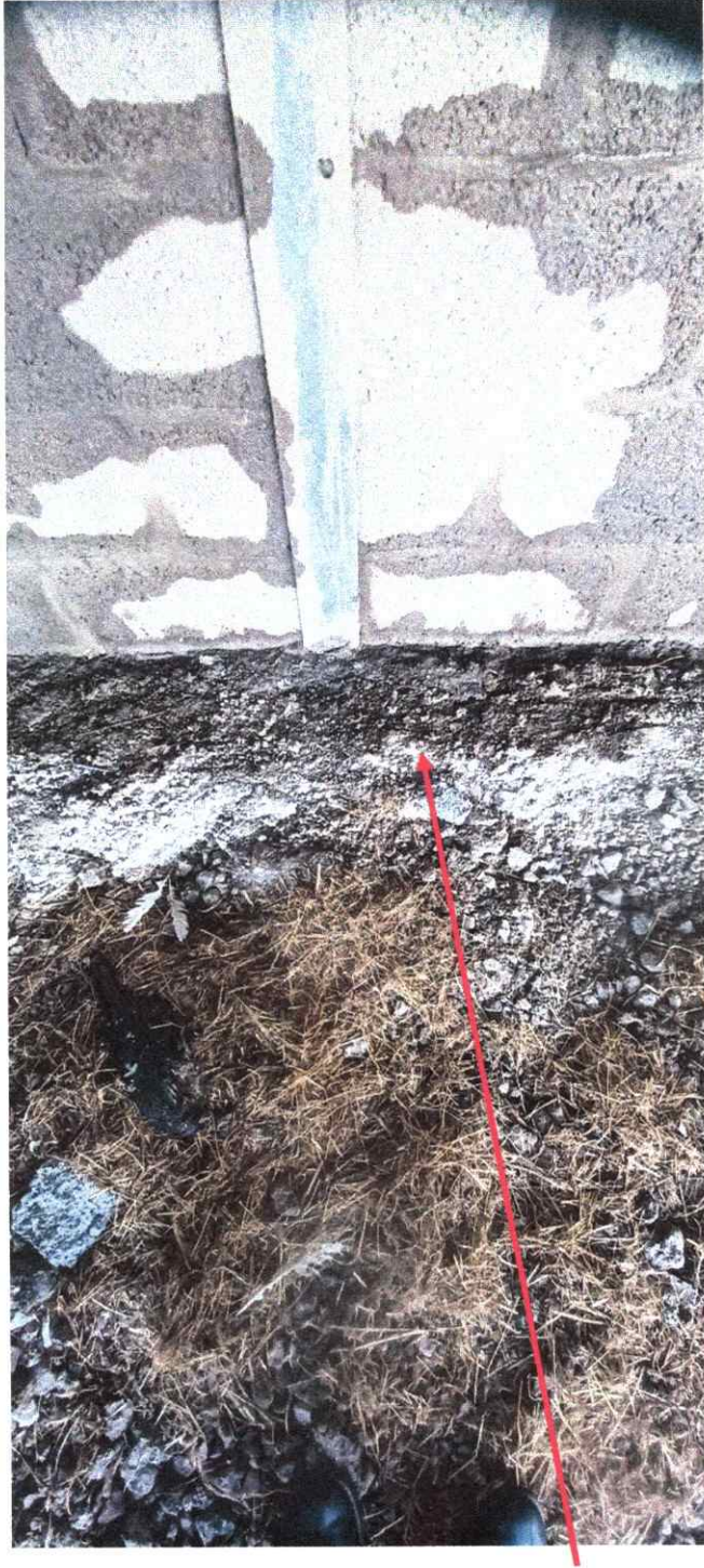
Foundation seen on rear south wall exposed at the surface which is found to be adequately sized to support a wall full height of the elevation.
