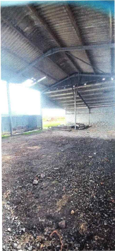
Internal photograph showing the lean-to structure to the east elevation. Also note the principal rafters which are in good condition.
