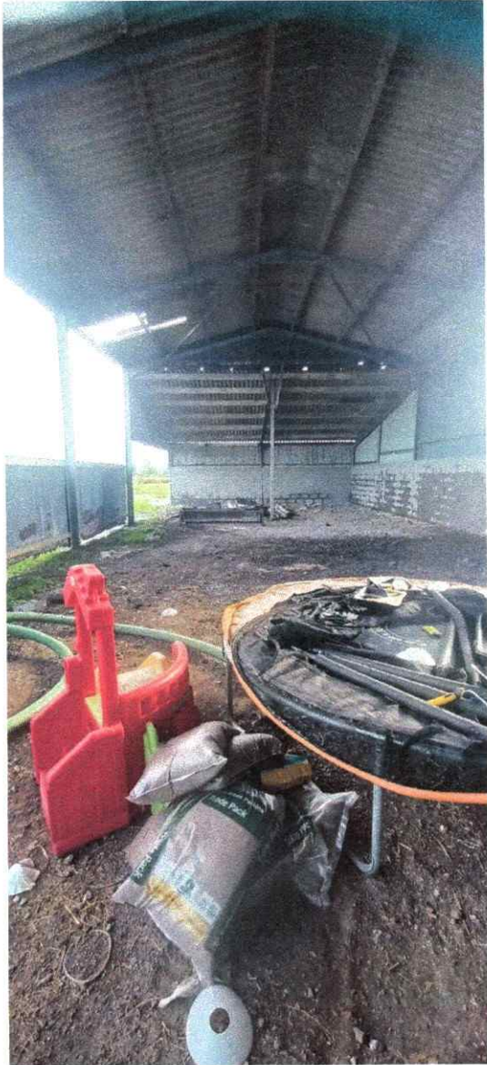
Looking towards the east elevation internally, showing the principal rafters and timber purlins which are in good condition.
