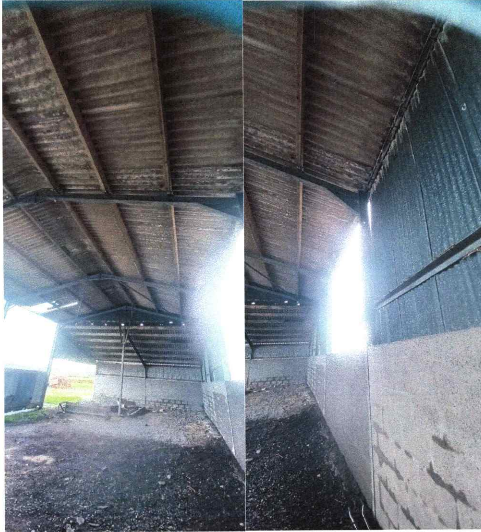
Photographs showing the internal structure and the rear south and east walls partly blocked adding lateral stability to the wall.
