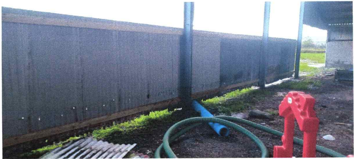
Front elevation facing north where the steel columns are exposed but nevertheless in good condition.
