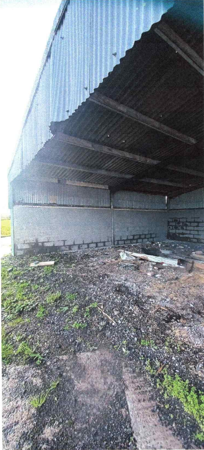
Front north elevation of the lean to located to the east of the barn.
