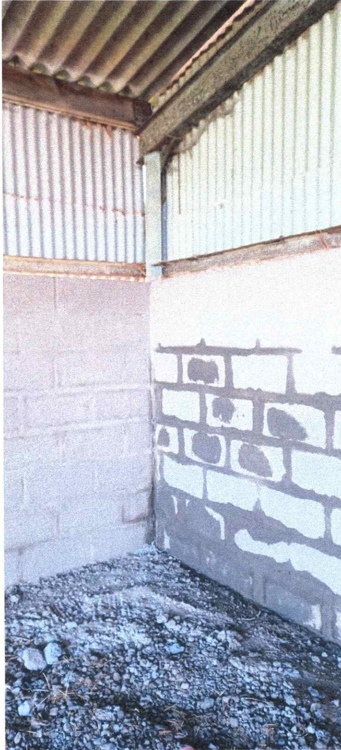
Photograph of southeast corner of lean to showing diagonal column, principal rafter and foundation which is evident at the surface.
