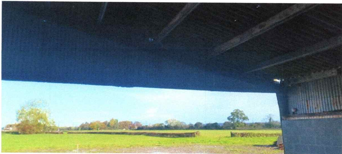
Photograph of timber purlins supporting lean to roof on east elevation which appear to be in reasonably good condition.
