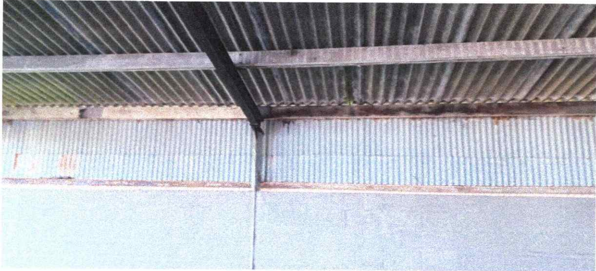
Photograph of diagonal column sections to the lean to on the east elevation supporting the principal rafters and timber purlins.
