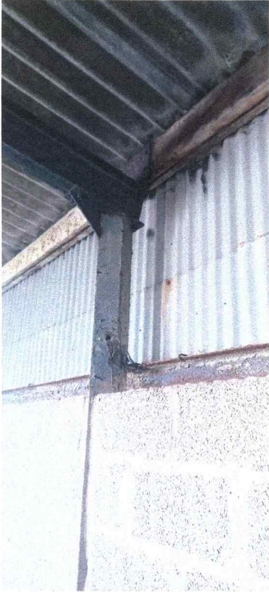
Diagonal steel sections used as columns to support the roof structure to the lean to on the east elevaton.
