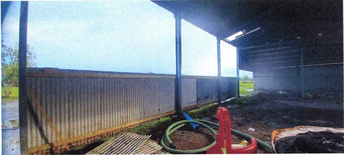
Internal view towards the north elevation which is partly open at the front.
