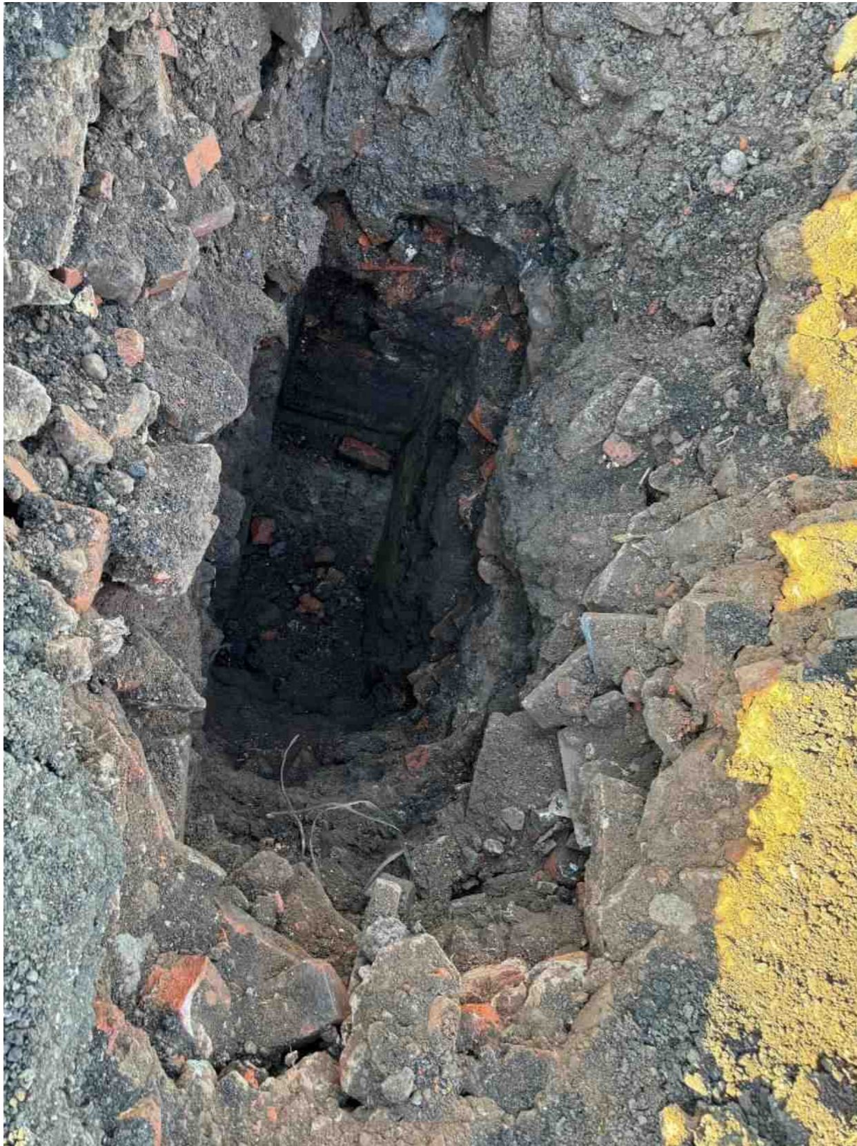
Photograph 2: Trial pit TP102 excavation – 2.60 m deep, brick fill to 1.80 m depth over 0.25 m ‘ash fill’ over ‘clay’
