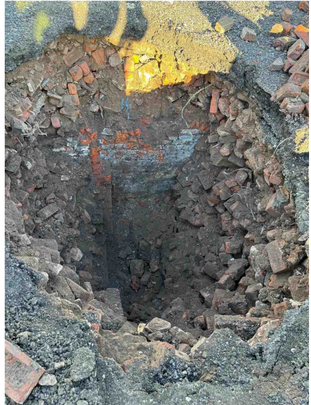
Photograph 3: Trial pit TP103 excavation – 3.00 m deep, brick fill to base with evidence of basement footings
