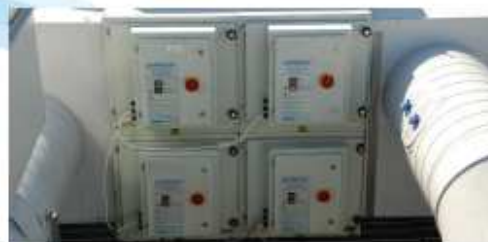
4 ESP Units Stacked in modular formation with a double pass
