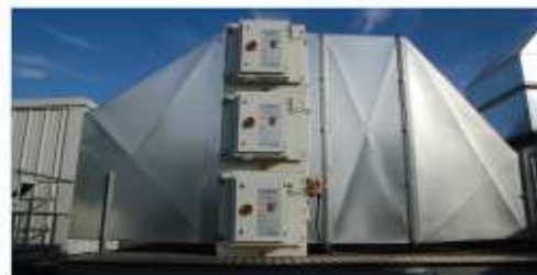
3 ESP Units Stacked in modular formation
