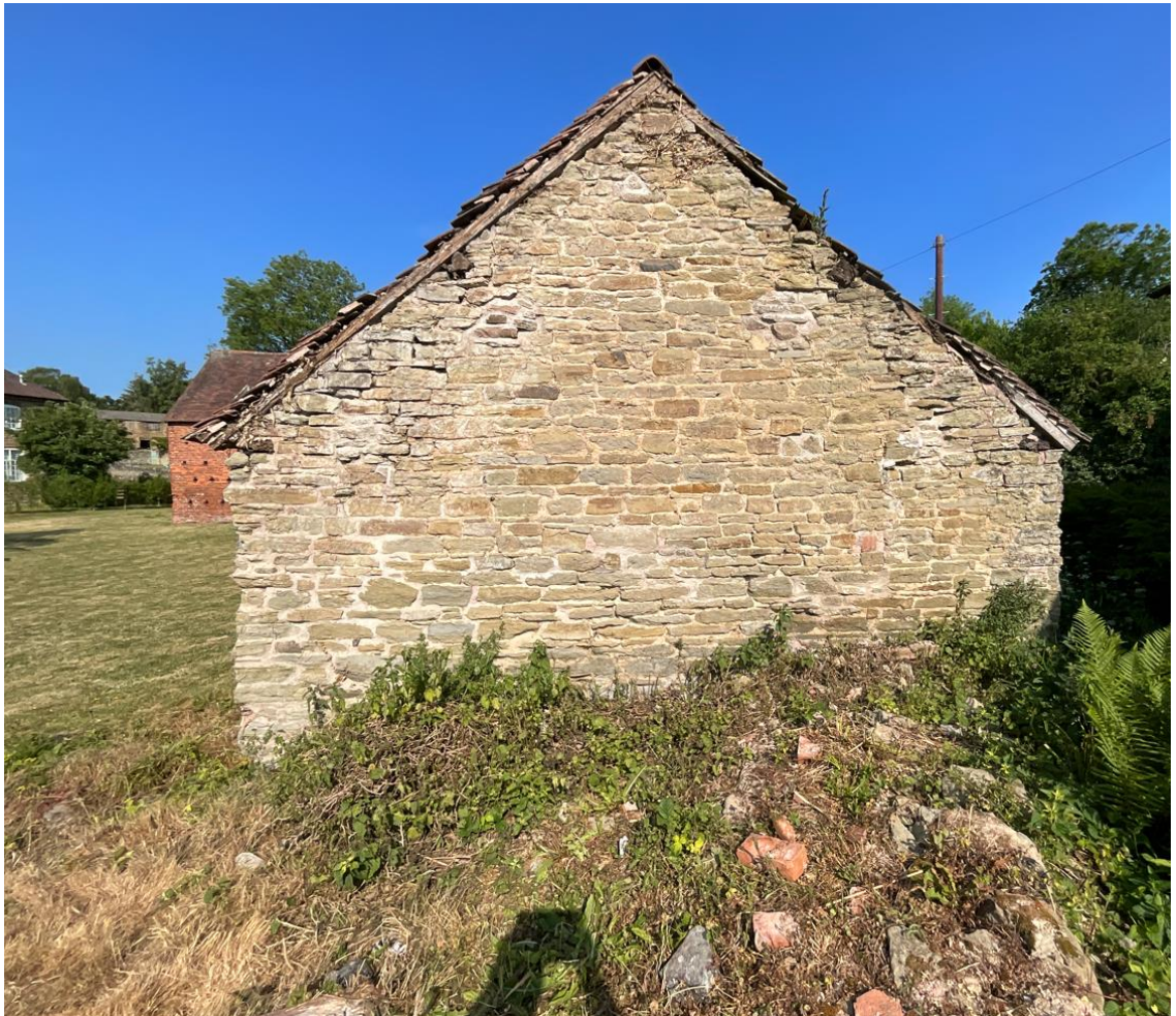
Plate 6 - Gable end of weather-boarded cattle shed showing evidence of once adjoining open fronted cattle shed purlin and ridge locations in the stonework now filled in.
