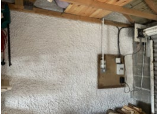
Picture 6 – Cable to run down the wall and new consumer unit to be fitted along side the Hybrid Inverter and Battery Storage
