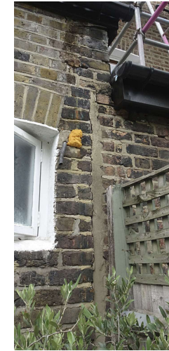
CONSTRUCTION Settlement. No independent flank wall to (9)
