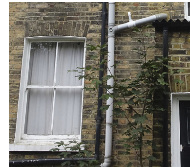
REAR ADDITION . VARIATION IN WIDTH Proximity of closet addition flank wall to window reveal
