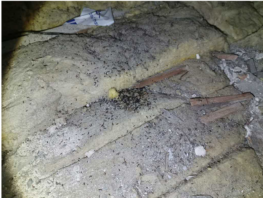
Figure 13: View of bat droppings within two-storey section.
