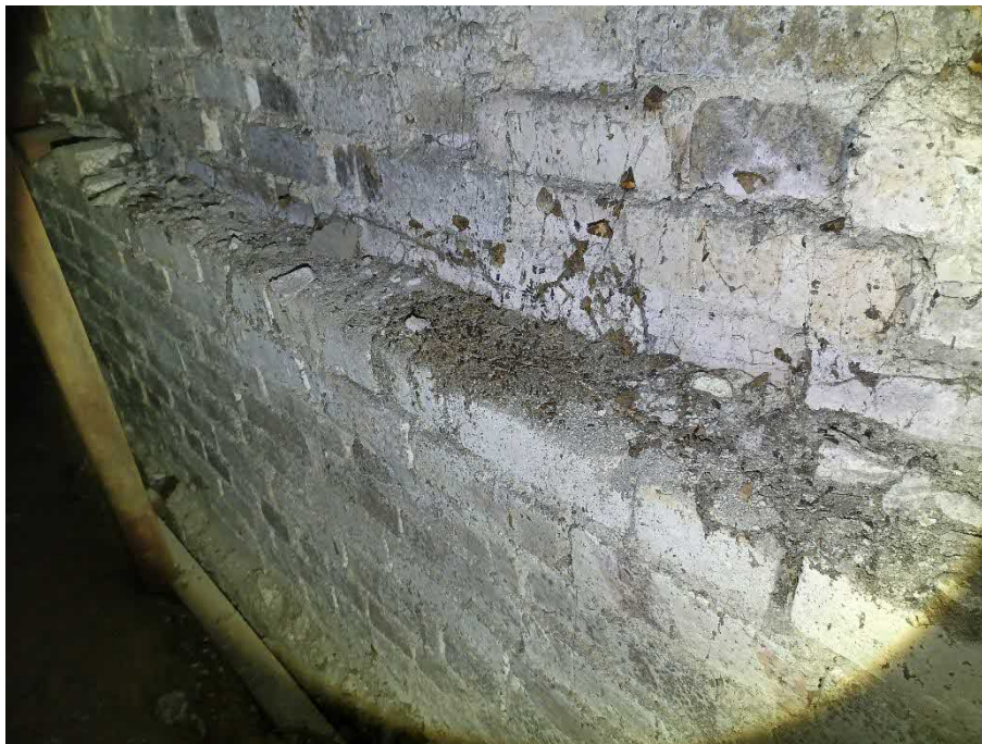
Figure 14: View of bat droppings and moth wings beneath the apex at the southern elevation of the two-storey section.
