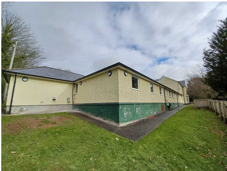
Figure 12: View of south elevation of single-storey extensions to the west of Meadowbrook House.
