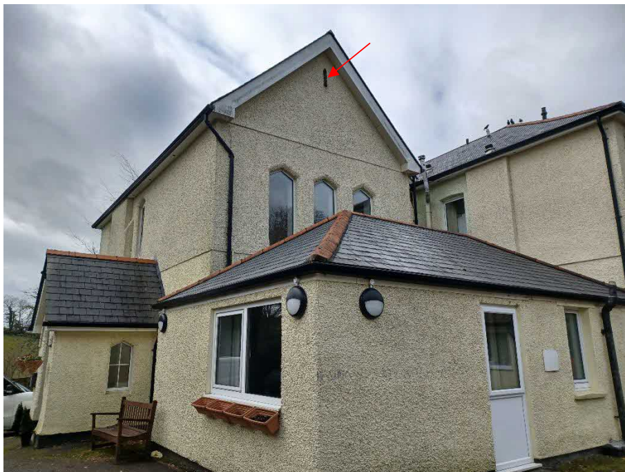
Figure 8: View of north elevation of two-storey section of Meadowbrook House, showing single-storey office in front; red arrow shows access into void.
