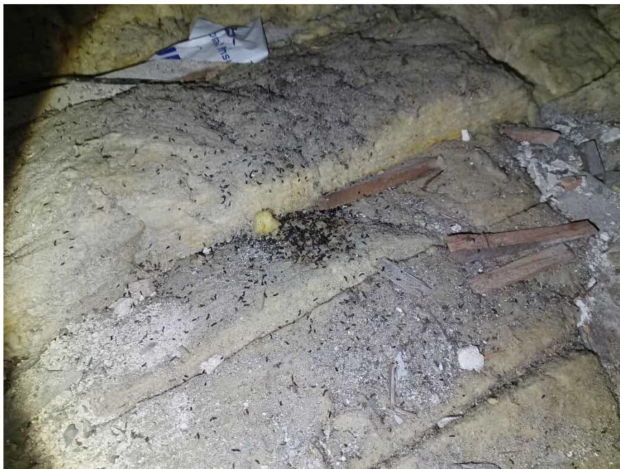
Figure 5: View of bat droppings within two-storey section.
