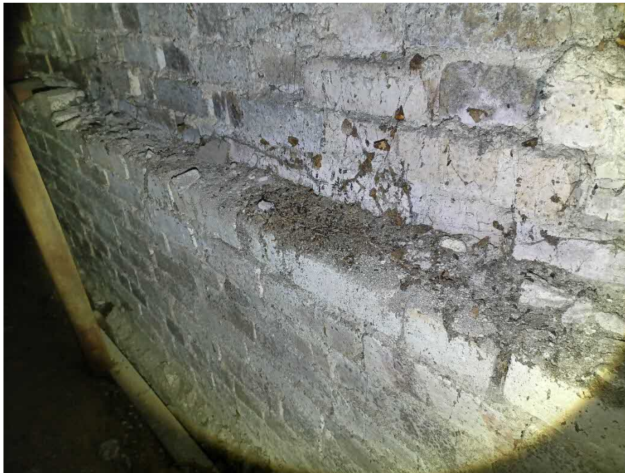
Figure 6: View of bat droppings and moth wings beneath the apex at the southern elevation of the two-storey section. DNA analysis confirmed the droppings to have been deposited by brown long-eared bat.
