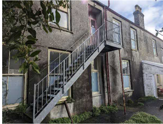
Photo 3. Showing the School Rooms from the south west and the external staircase
