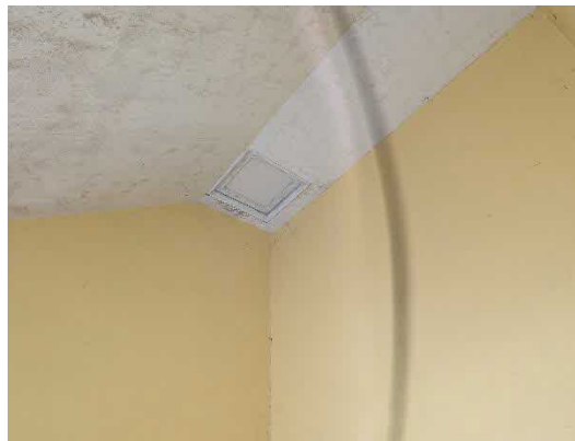
Photo 8. Showing the partially vaulted ceiling and small roof void above the room and stairwell at the eastern end of the building on the 1 st floor
