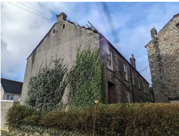
Photo 1. Showing the School Rooms from the north east with the northern elevation and eastern gable end being in view
