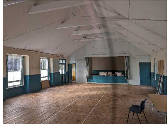
Photo 7. Showing the large room at the western end of the 1 st floor
