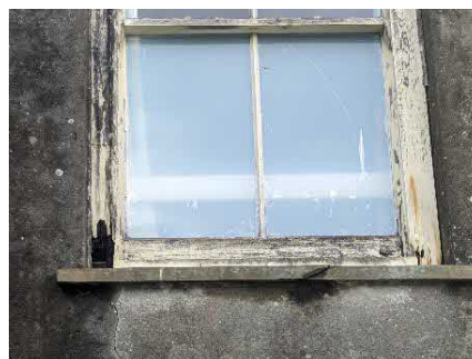
Photo 9. Showing the hole in the base of the sash window
