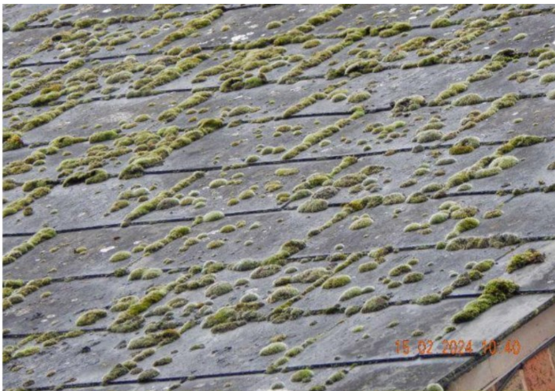
Image 4 – Close view of the main roof coverings to demonstrate example of condition
