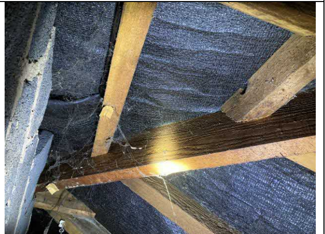
Photo 4 Cobwebbed roof timbers
