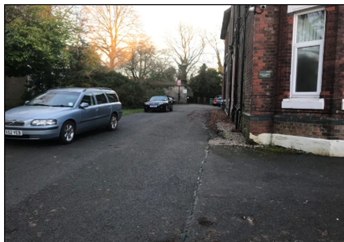
Plate HTN3 - Internal site driveway arrangements and additional hardstanding strip to side of building.
