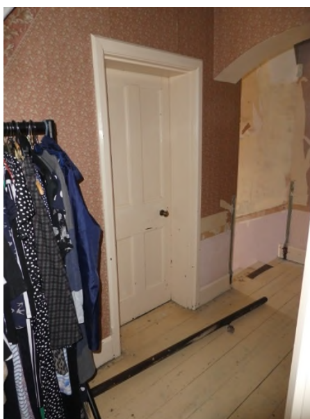
Figure 51: Cupboard door at the top of the stairs
