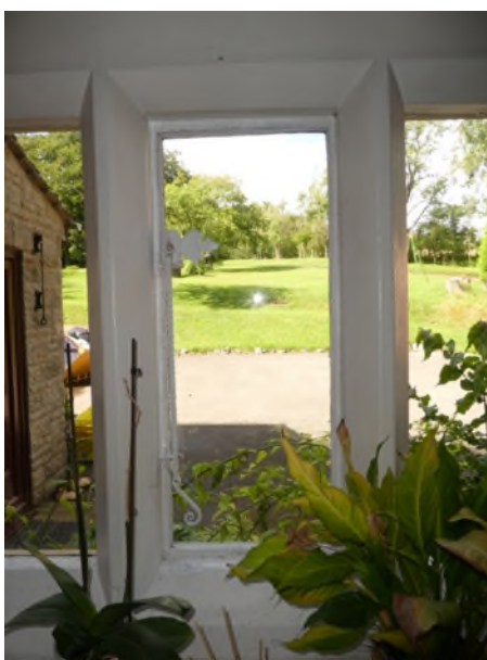
Figure 32: Detail of a side opening iron casement in the window on the north side of the kitchen
