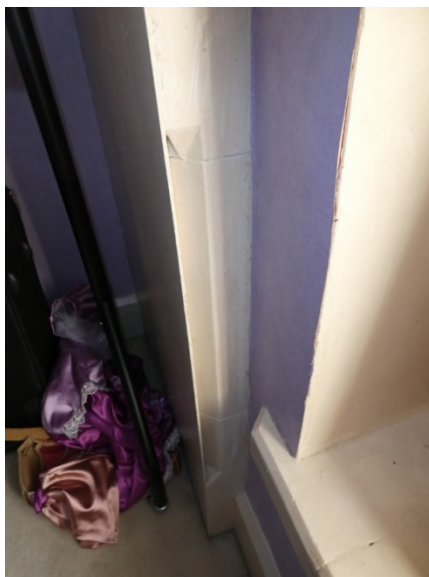
Figure 50: Detail of a chamfer and stops on the right hand side of the blocked fireplace
